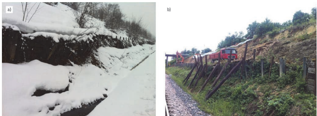
Figure 2. Degradation of implemented remediation measures: a) completely deformed prefabricated concrete wall; b) makeshift slope protection structure
