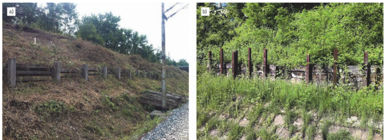
Figure 1. Remediation by: a) prefabricated concrete wall; b) wall made of driven rails and wooden sleepers
